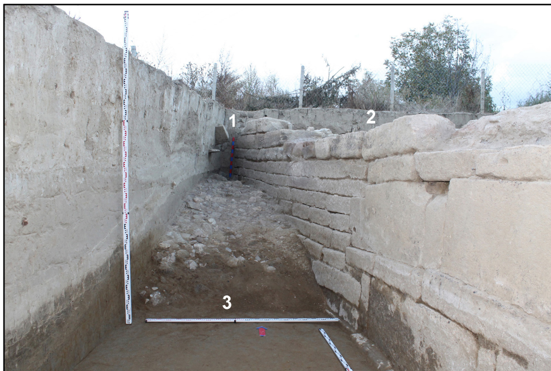
Fig. 6. The Rubas Fortification of the 6th c. 1 – Wall 2, western facade, northern section; 2 – Wall 2, western facade, central section; 3 – mudflow deposits. View from the south. Photo of 2017
